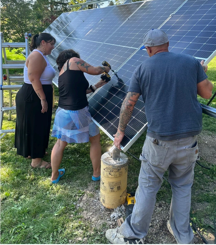
Audrey Huntley from No More Silence, Serena Mendizabal from Sacred Earth Solar, and solar installer Mike from Solar Associates installing the solar panels for the Hummingbird Lodge. Photo credit: Audrey Huntley, Fall 2023
